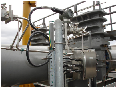
A dual run Senior orifice fitting installation.
