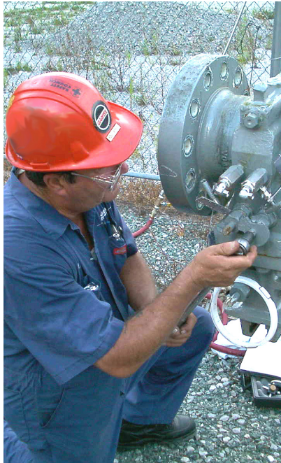
Proper maintenance of orifice fittings helps minimize lost and unaccounted for gas.
